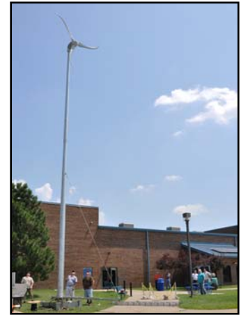
Workers lift a new wind turbine at the Southwestern Illinois College Sam Wolf Granite City Campus recently. The wind turbine was installed to both power the campus, provide additional power back into the electricity grid and provide students in college sustainability courses with a real-world example of the technology they will be studying.
